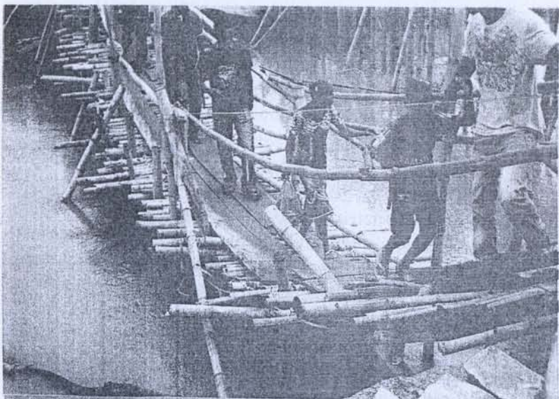
Plate 3: A make-shift bamboo foot-bridge constructed by Apete residents to facilitate movement of children and adults from Apete to the rest of the Ibadan city after the concrete bridge on Ona River was swept away by the flood of 26 August, 2011. See the state of fear in the children as they are being assisted to walk on the foot-bridge.
