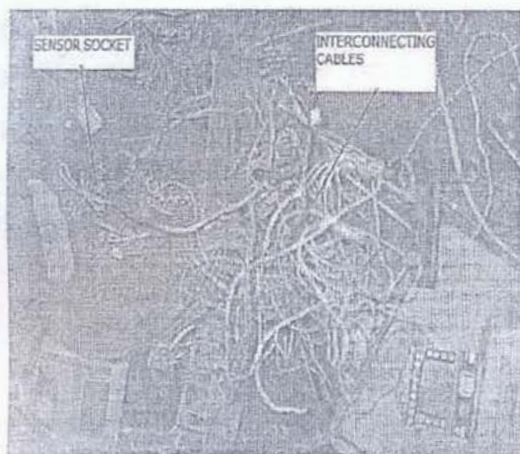
Figure 5: Picture Showing Interconnection of some Hardware Components
