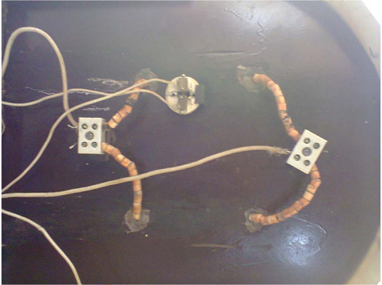
Figure 3.15 Furnace Rear View
