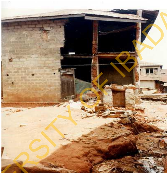
This picture demonstrates lack of access to effective sewage system.
